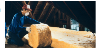
Figure 3. Insulation being installed. Learn how to hire a qualified professional or steps to do it yourself at www.energystar.gov/campaign/seal_insulate/identify_problems_you_want_fix/div_checks_inspections
