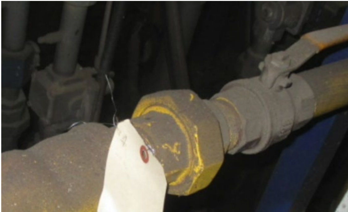
Photograph of leak
