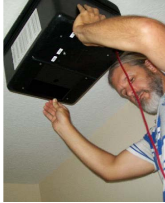
Bathroom Exhaust: Exhaust fan flow box.
