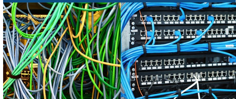
Above: (Left) Example of bad cabling in a data center, (Right) an example of good cabling.
