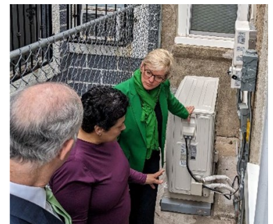
Photo caption: Senator Casey, Secretary Granholm, and Nancy with her new heat pump and rooftop solar system.
