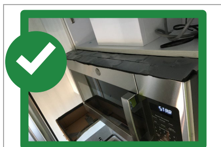
Figure 4: An example of a neoprene cover used to block a secondary intake on the top of a microwave exhaust and direct all intake air to the underside of the microwave. (Duct mastic tape is also commonly used.) This practice provides the rater with the maximum possible flow tested through a single location.
