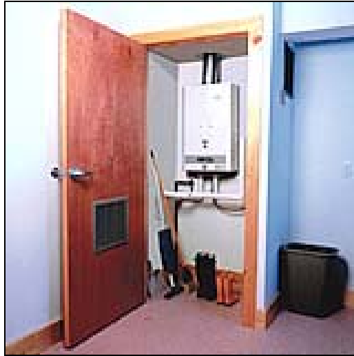
Figure 2-1 Whole-House Installation of Gas Tankless Water Heater (Illustration courtesy of Controlled Energy Corp.)
