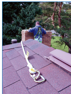
Figure 7: Roof anchor should be installed on a roof subsurface or vertical wall.
