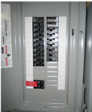
Figure 10: 70-Amp Double Pole Breaker. The electric service panel should have designated and labeled slots suitable for a 70-amp double pole breaker for use by the solar PV system.
