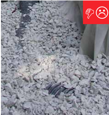
A. The drain tile is not wrapped in fabric and could become clogged with debris.
