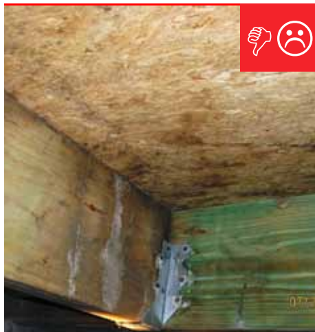
C. Building materials have signs of water damage and high moisture content.
