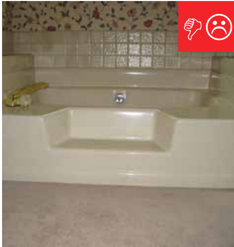
A. There is carpet installed too close to the plumbing fixtures in the bathroom.
