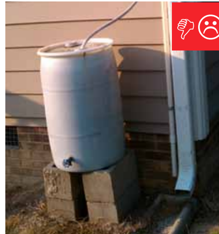
D. Rain barrel installed without an overflow spout that terminates away from foundation.
