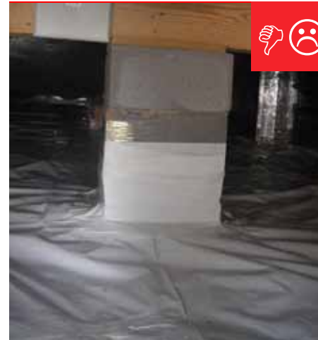
C. The polyethylene sheeting is not staked or attached to furring strips for mechanical support.
