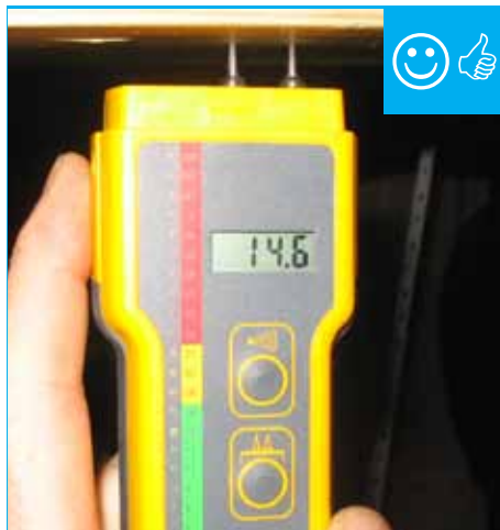
A moisture meter verifies that the moisture content of the framing is below the recommended 18%.
