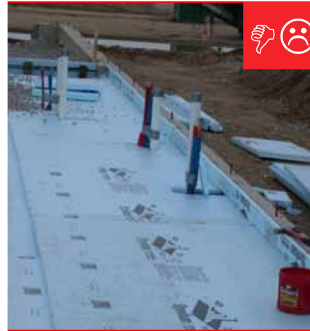
C. The seams of the rigid insulation are not taped and it will not provide a complete capillary break.
