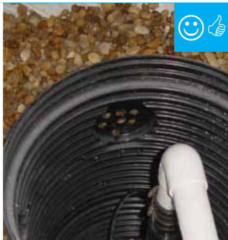
The drain tile connects to a sump pump which will pump water away from the foundation.
