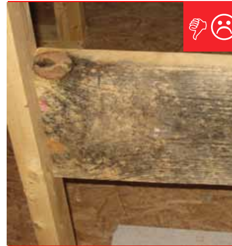
B. Building materials with visible signs of mold have been used.
