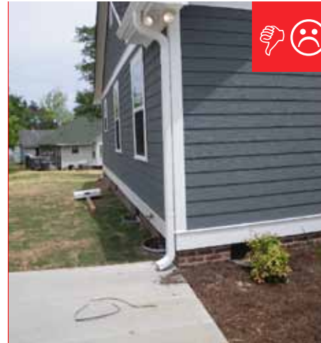
B. The downspout terminates too close to the foundation of the house.
