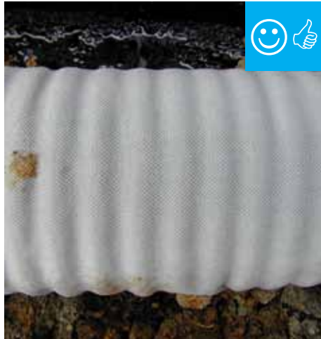
The drain tile is wrapped in fabric which will prevent it clogging with debris.
