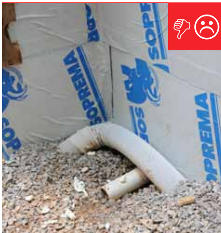
C. The drain tile is not installed to terminate properly and will not transport water to the exterior.
