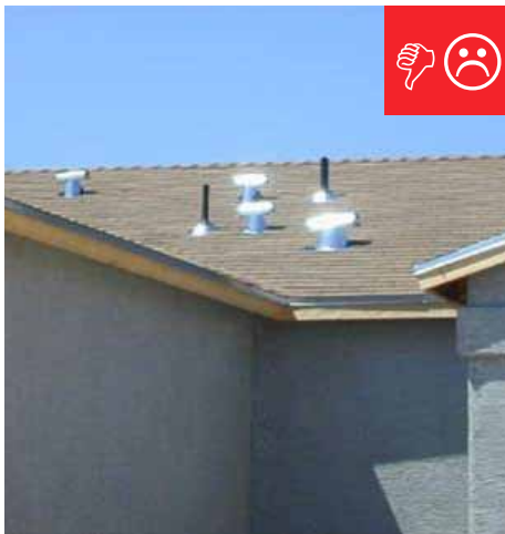
C. Ventilation inlet is too close to exhaust outlets and does not extend at least 2 ft. above the roof deck.
