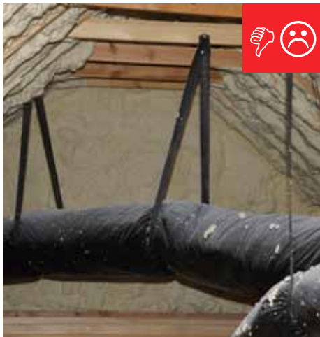
C. Straps are spaced too far apart causing the straps to compress the duct under its own weight.
