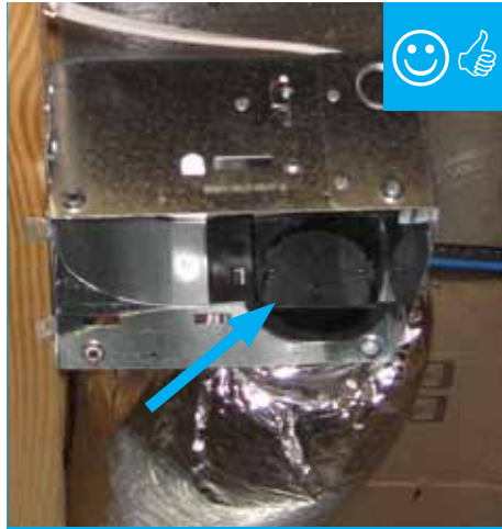
Fan shares exhaust and has a back-draft damper installed.
