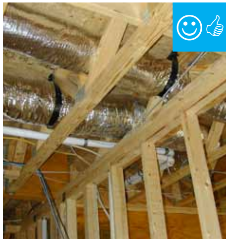
Ducts well supported by framing and straps as needed.
