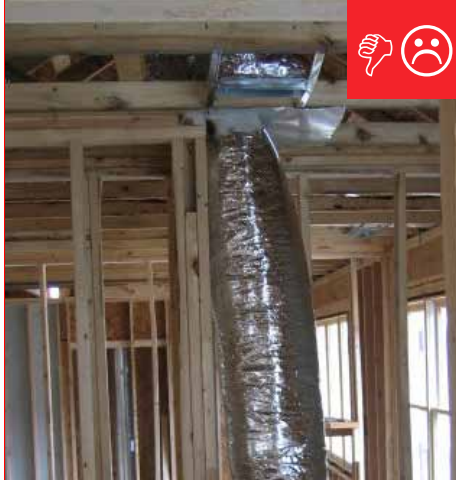
A. Duct is compressed.
