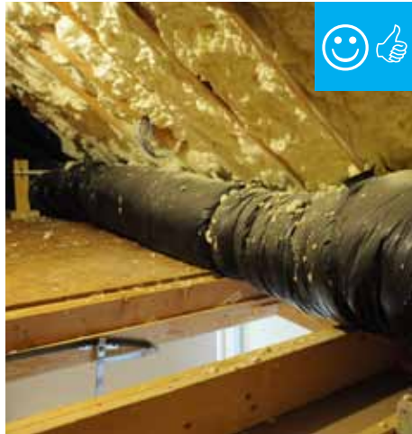
Duct is run straight and supported properly.
