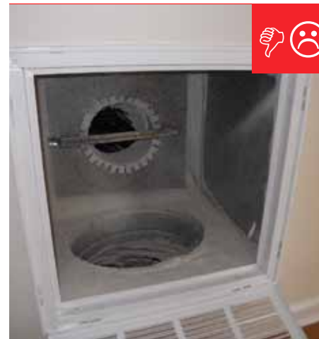
D. There is no filter installed to filter the outdoor air.
