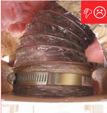
A. Connection in place but not sealed.
