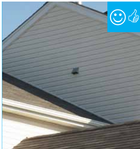
Ventilation inlet is not near any exhaust outlets/contamination sources and is at least 2 ft. above the roof deck.
