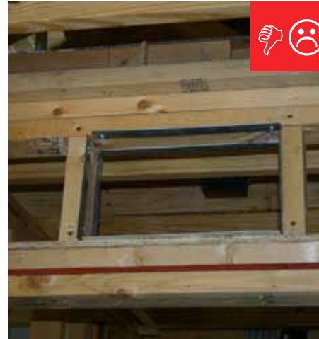
B. Transfer grill not sealed.
