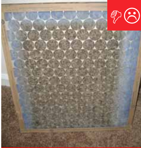
A. The installed filter is not a MERV 6 filter.
