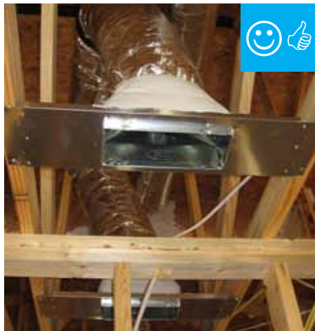
Duct to boot connection of jump duct is properly sealed with mastic.
