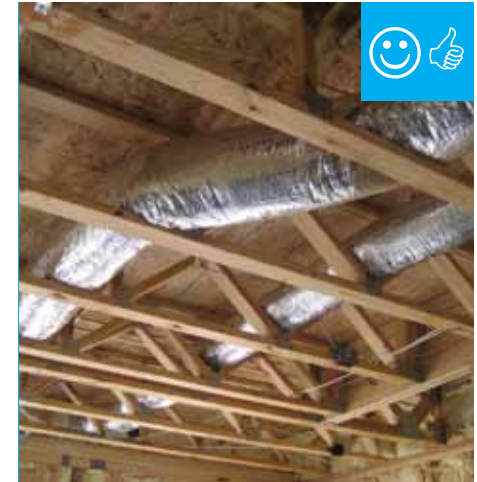
Ducts are run straight and supported properly.
