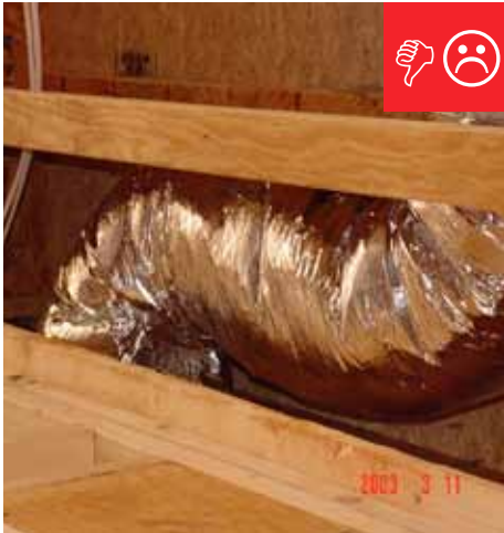
A. Duct is kinked in cavity.
