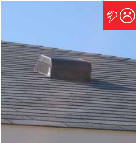
B. Ventilation inlet does not terminate high enough above the roof deck.
