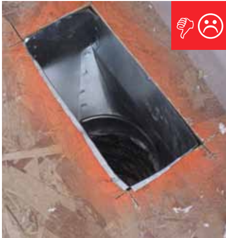
A. Boot to floor connection not sealed.
