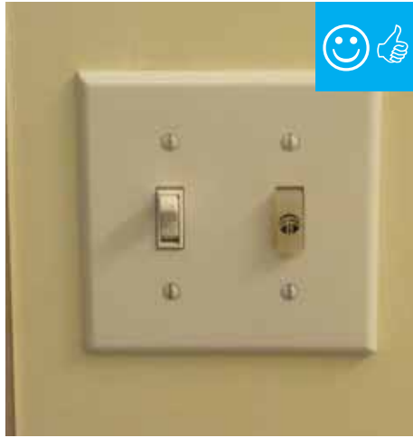
Manufacturer labeled ventilation switch.
