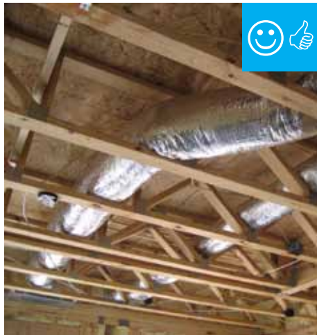
Ducts properly installed without compression and appropriately supported.
