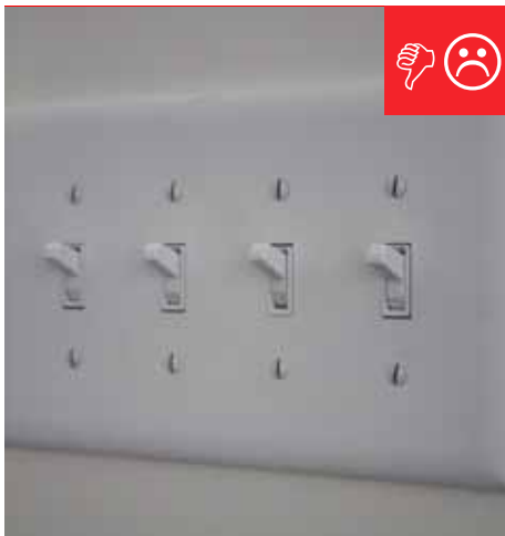
B. Ventilation control is not obvious.
