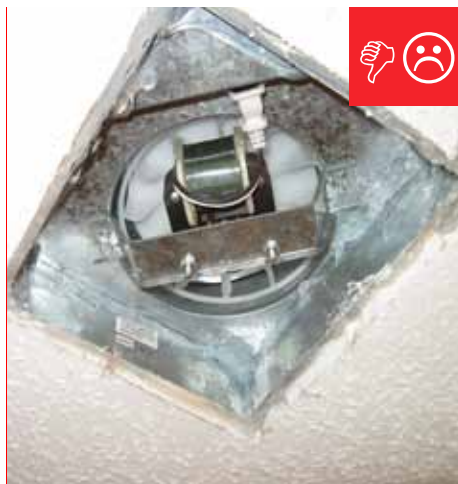
D./E. The fan does not have an ENERGY STAR label.
