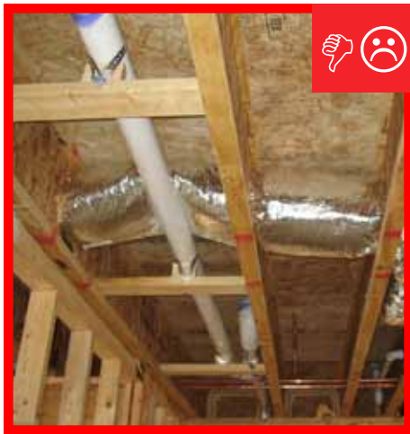
A. Duct is compressed.
