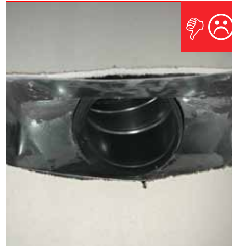
A. Boot to drywall connection not sealed.
