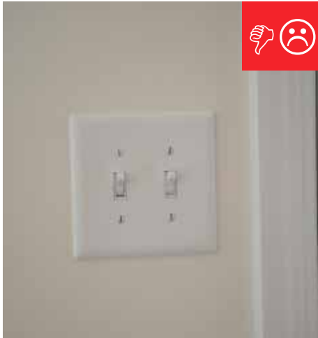
A. Ventilation control is not obvious.
