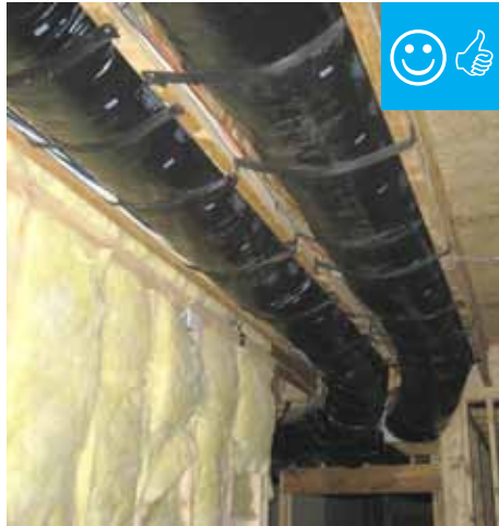
Ducts well supported.
