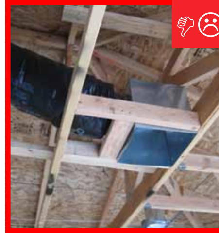
B. Return box has not been sealed.
