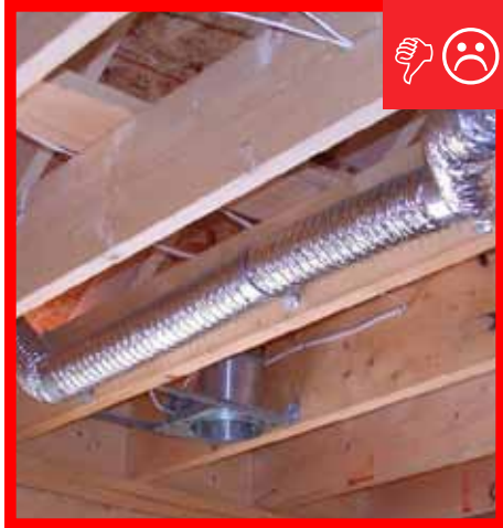
A. Duct is located in unconditioned space and is not insulated.
