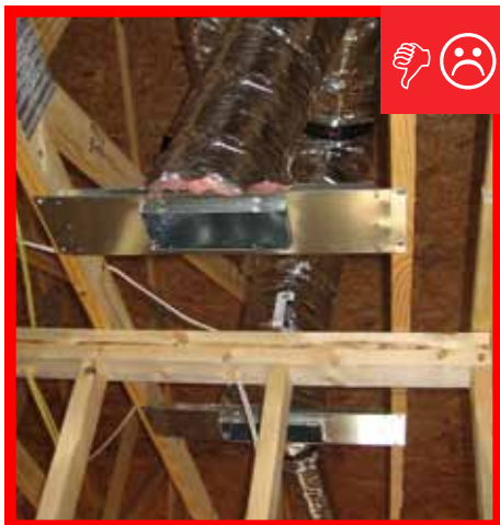
C. Duct to boot connection of jump duct not fastened and sealed.
