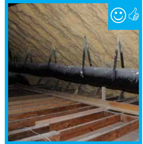
Ducts well supported.
