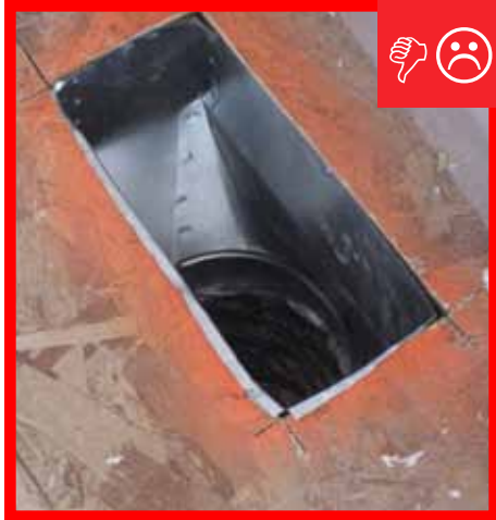
A. Boot to floor connection not sealed.
