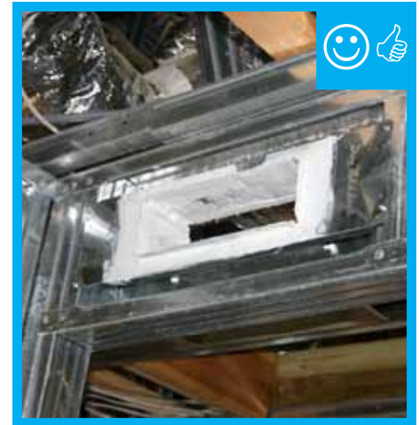
Transfer grill sealed with mastic.
