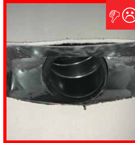
A. Boot to drywall connection not sealed.
