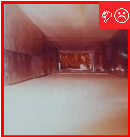
D. Cavity was not air sealed.
