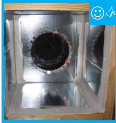
Return duct has been properly sealed with mastic.
