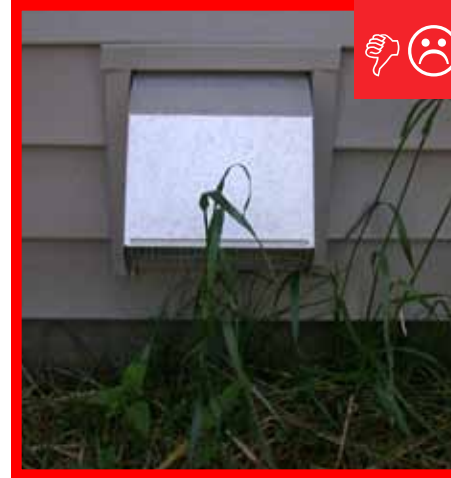
C. Ventilation inlet is too close to the ground and is being blocked by the grass.
