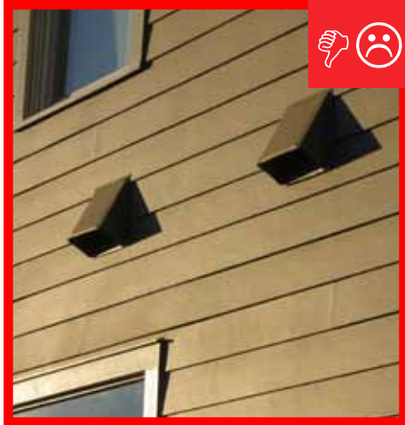
B. Ventilation air inlet is too close to exhaust outlet.
