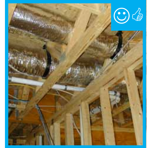
Ducts properly installed without compression and appropriately supported.
