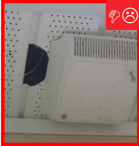
A. Exhaust terminates inside of soffit and was just covered.
