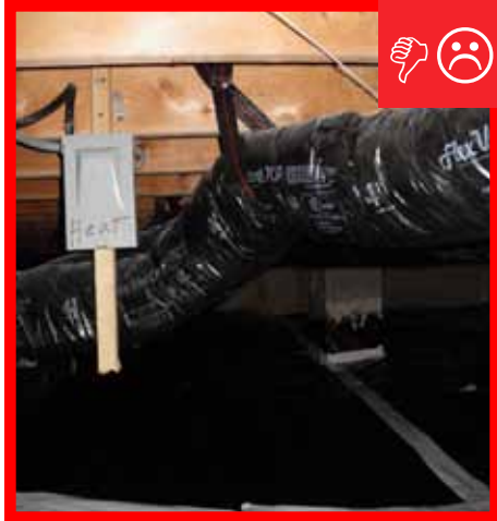
A. Duct sagging because supports not installed at regular intervals.
