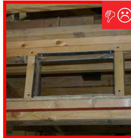
B. Transfer grill not sealed.
