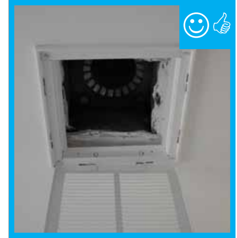
Return box has been properly sealed with mastic.
