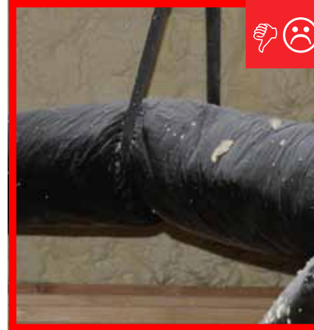
B. Duct is insulated but strapping is compressing the insulation therefore reducing the R-value.
