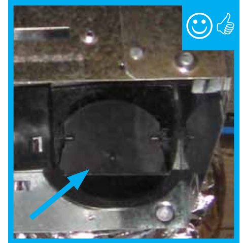
Packing tape has been removed and damper will be able to function properly once fan is installed.
