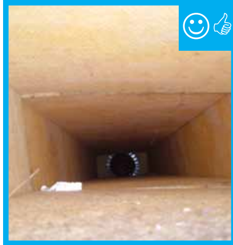
Cavity used for duct has been lined with rigid insulation and is ready to be air sealed.
