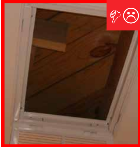
B. Cavity used for return is not insulated and is not air sealed, which will pull in air from outside.
