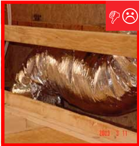
A. Duct is kinked in cavity.
