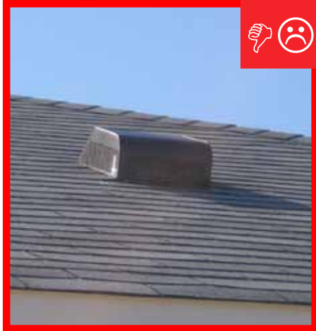
B. Ventilation inlet does not terminate high enough above the roof deck.
