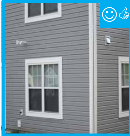
Ventilation inlet is greater than 10 ft. from known contamination source.
