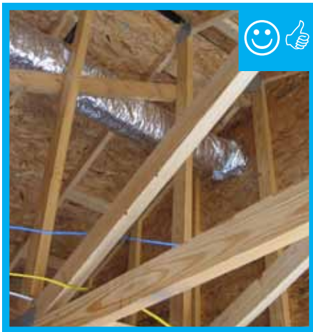
Exhaust duct is well supported by framing and support straps.
