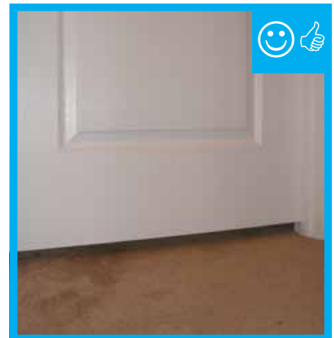
Door has been undercut to allow for specified amount of air flow therefore contributing to pressure balancing.
