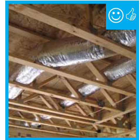
Ducts are run straight and supported properly.
