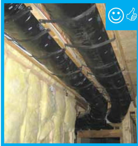
Ducts well supported.
