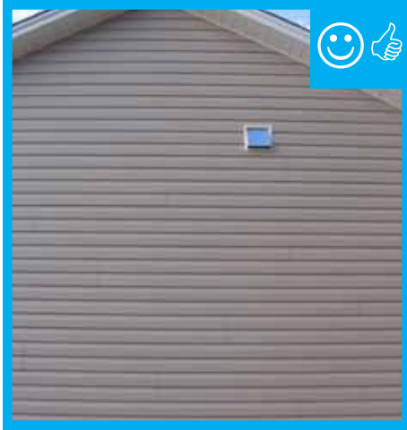
Exhaust terminates to the outside away from air inlets.
