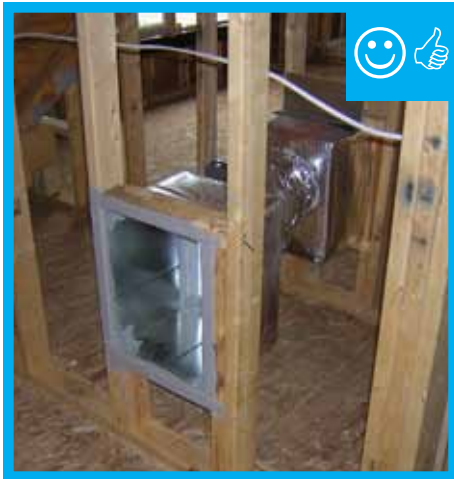
A. Grill and duct size based on calculated requirements for net free area.
