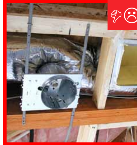
A. Recessed can light is compressing duct work.
