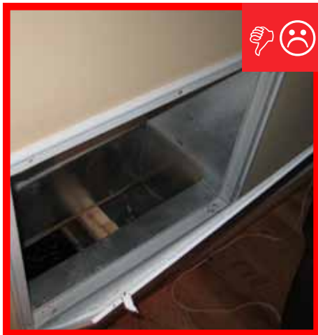
C. There is no filter installed in the HVAC system.
