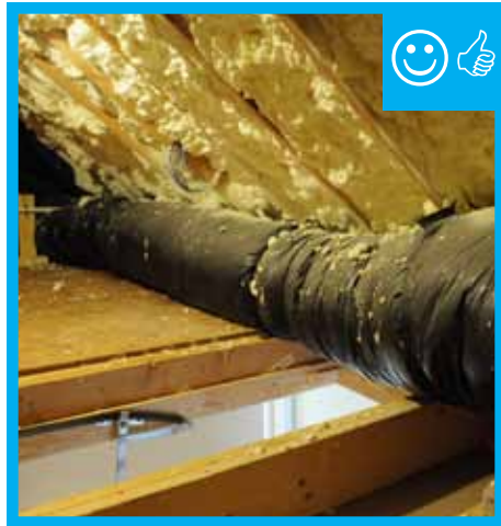
Duct is run straight and supported properly.
