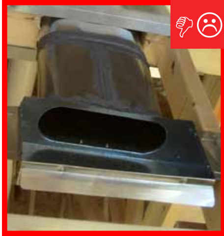
A. Return has not been sealed.
