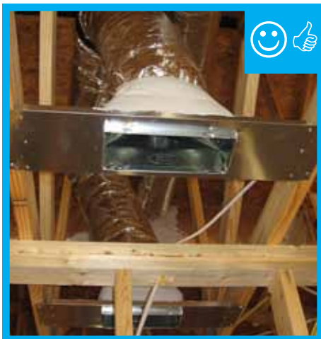
Duct to boot connection of jump duct is properly sealed with mastic.
