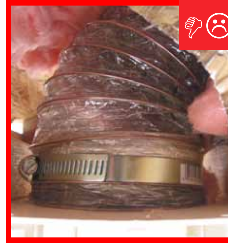
B. Exhaust duct only mechanically fastened and not sealed.
