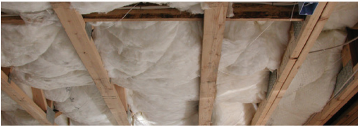
Insulation has misalignment, compression, and gaps.
