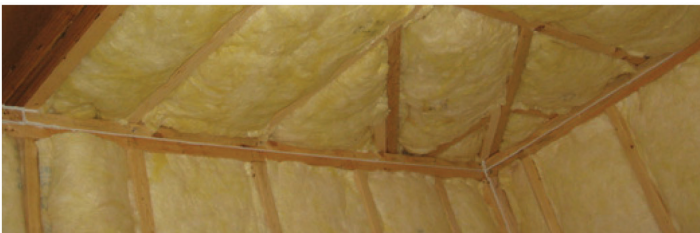
Insulation is fully aligned with air barrier with no major compressions or gaps.
