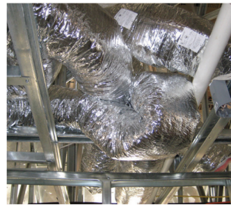
Ducts are crammed into cavity, kinked and sharply bent.
