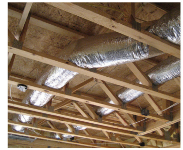
Ducts are run straight and supported properly.
